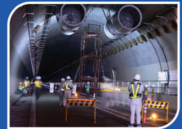
Lighting system, Dust collector and Fan ventilation system for tunnel
