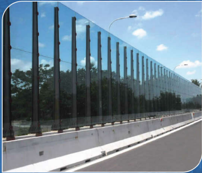
Noise barrier system
